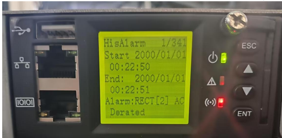
Figure 3-12 Historical alarm information screen
