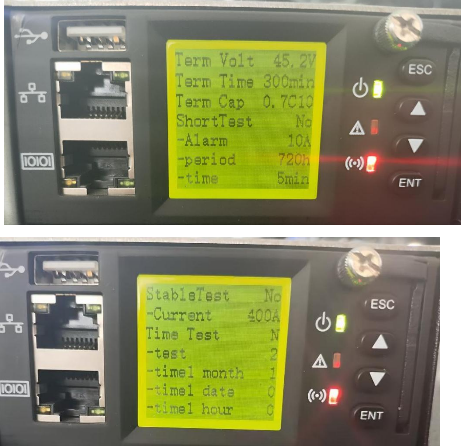
Figure 3 -21 Battery test parameter setting screen
