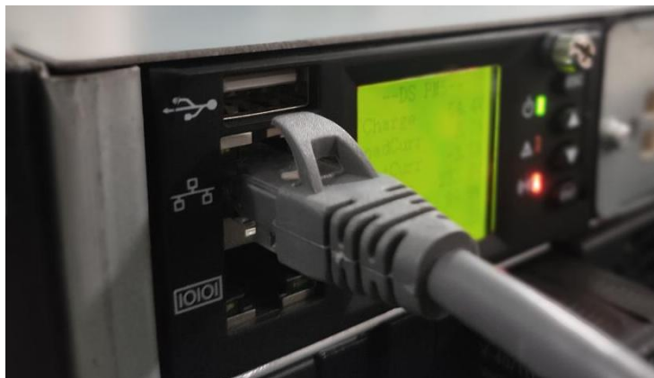
Figure 4-2 Monitoring network cable connection
