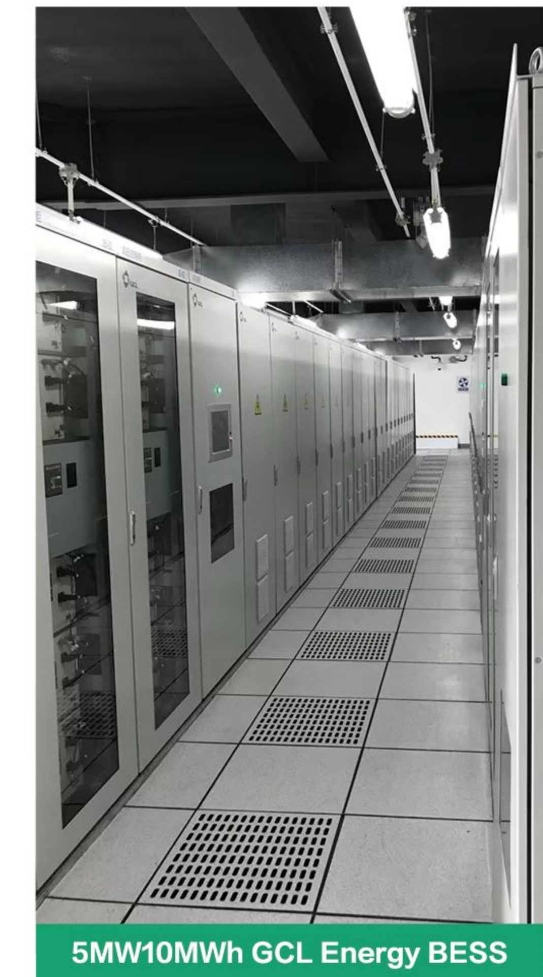
5MW10MWh GCL Energy BESS
