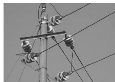
Dead-end for AAC conductor
